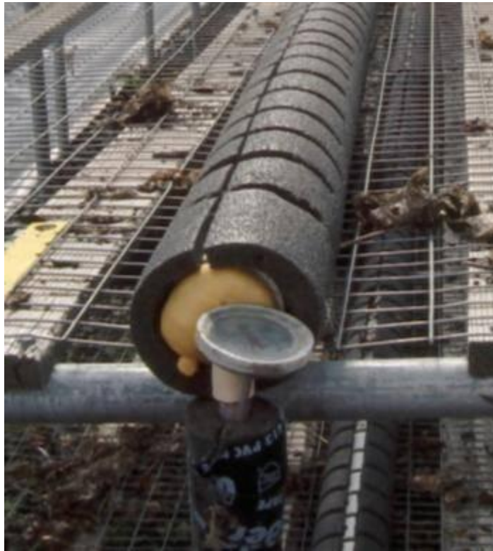
Photo of a hot-pipe system showing a heating pipe wrapped with insulation.
